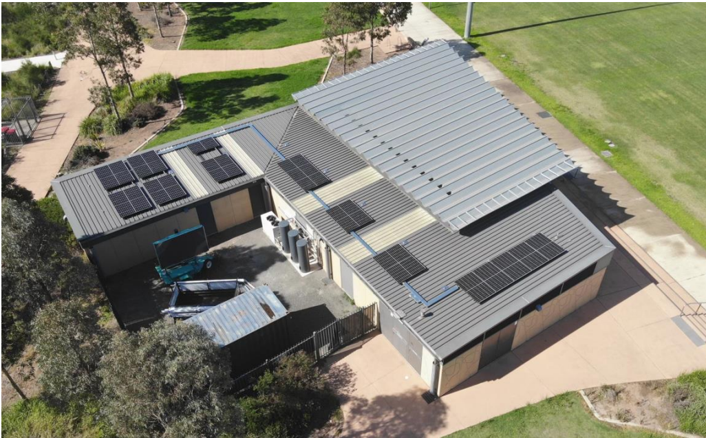
Aerial view of installed rooftop solar system (10kW) and three heat pump hot water systems at Jack Brabham Reserve as part of Council's first electrification projects.
