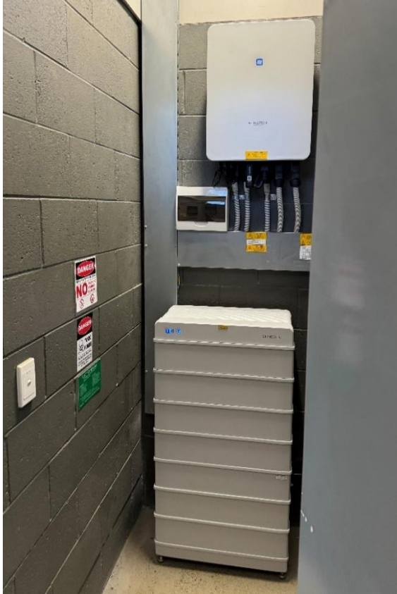
Installed 20kWh battery at Jack Brabham Reserve amenities building – Camden Council's first battery system providing additional resilience for the local community.
